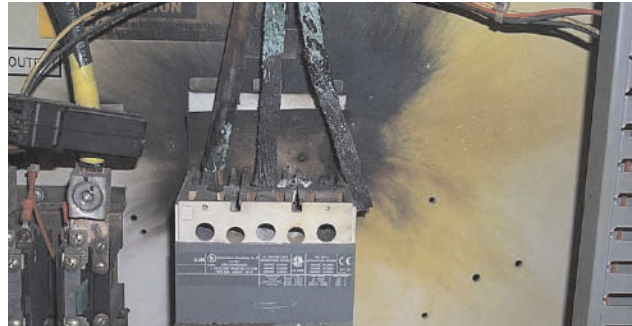
Photo 3, Arcing Caused by Loose Input Contacts
