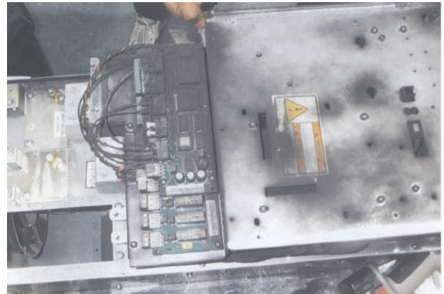
Photo 1, Fan Injecting Dust into Drive Enclosure
